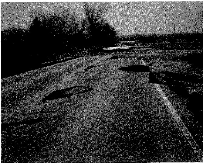
Flood damage north of Morse Bluff, 1978
